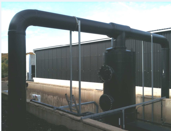
Acid scrubber at the demonstration facility in Fridhaff, Luxembourg.
